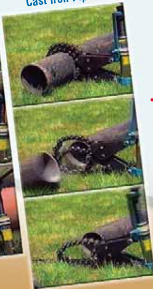
Cast Iron Pipe
