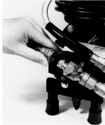
Figure 2 – Connect Water Supply Hose to Jetter. Close Inlet Supply Valve (shown in closed position.)
