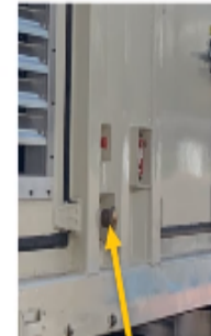
Fire Department Connection
