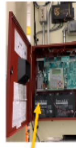
Fire Control Panel
