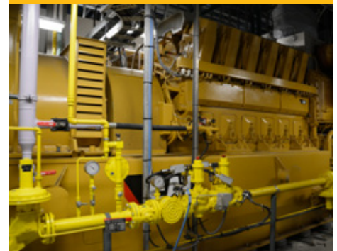
Cat® CG260-12 natural gas generator set installed at Markham District Energy's Birchmount Energy Centre for its combined heat and power (CHP) application.
