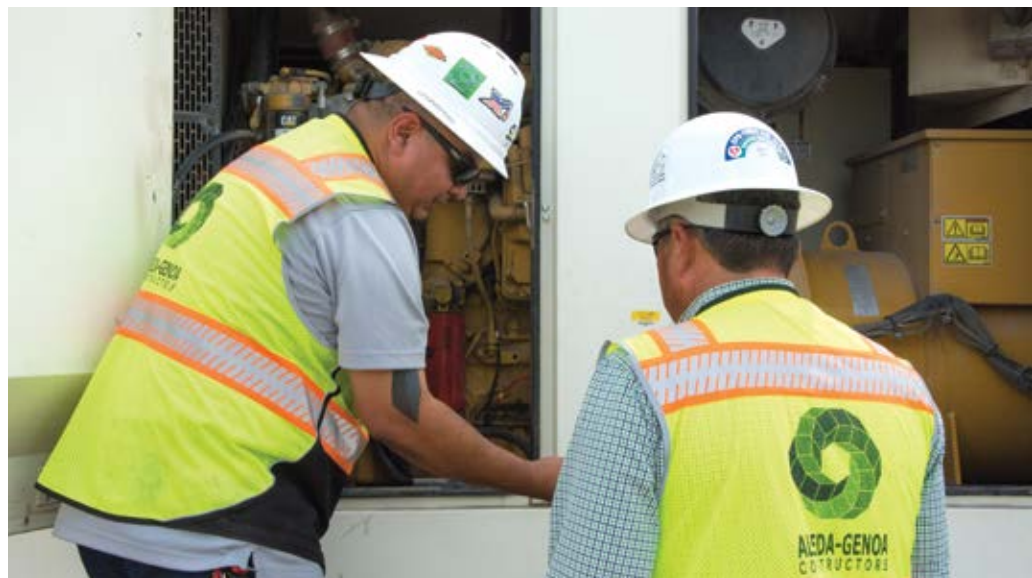
Junior Medrano and Rene Sanchez of Almeda-Genoa Constructors inspect a rental power generator set provided by ERS Cat.
